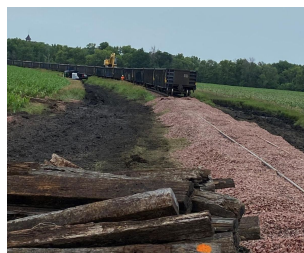
D & I operating crews, LGE Maintenance of Way, Herzog and Niewohner Construction working together to begin the recovery process.
